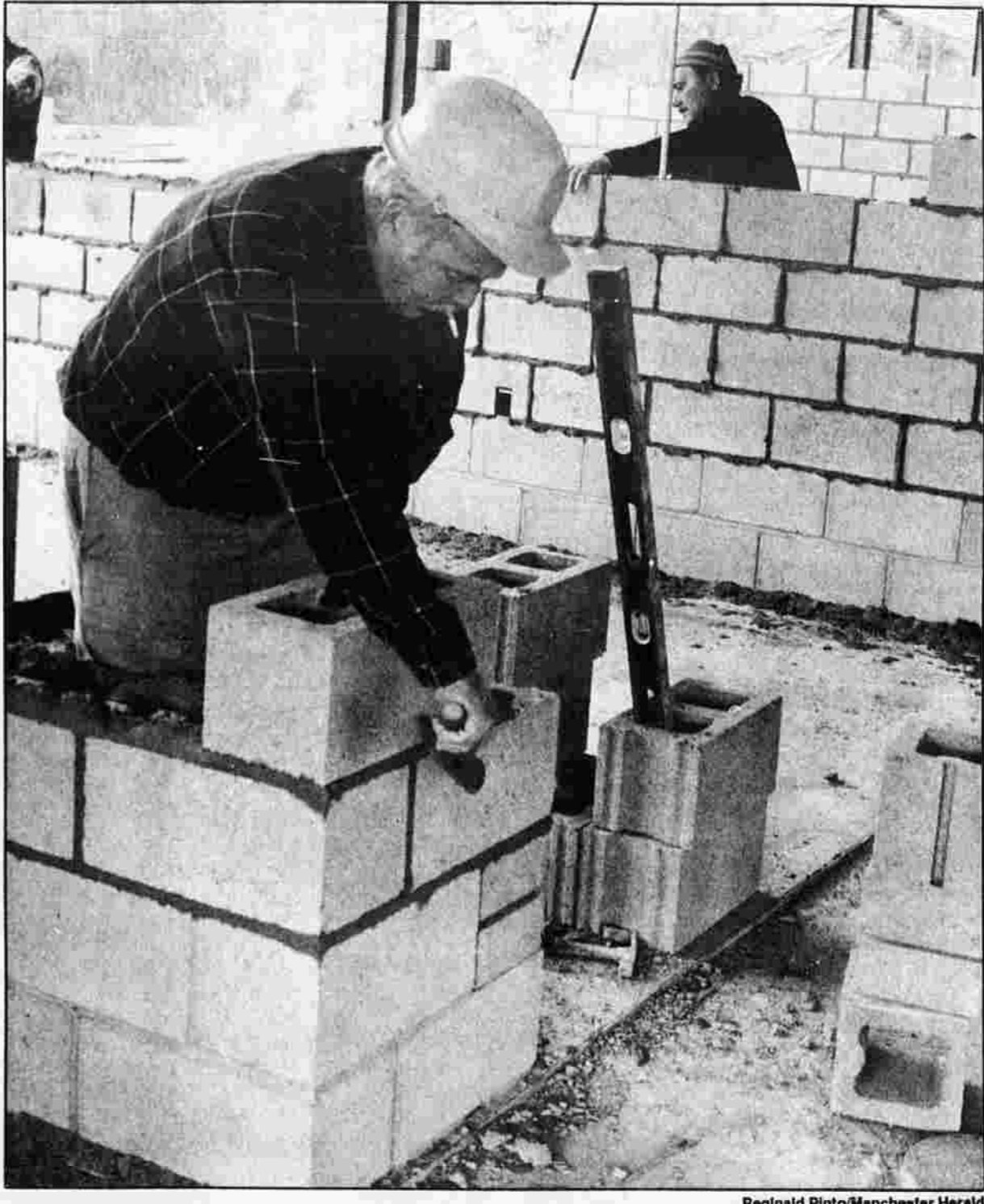
LAYING BLOCKS — Richard Bradshaw, foreground, of Middletown, and Salvatore D'Agostino of West Hartford, of GMC Masonry Construction of Hartford, lay concrete blocks for the new post office on Sheldon Road in Manchester.
